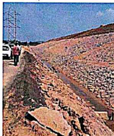
Figure 12: Deposition of soil in rocktoe at Ch 18.85 km (tank bed portion)
