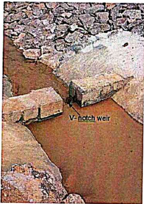
Figure 3: V-notch weir in toe drain
